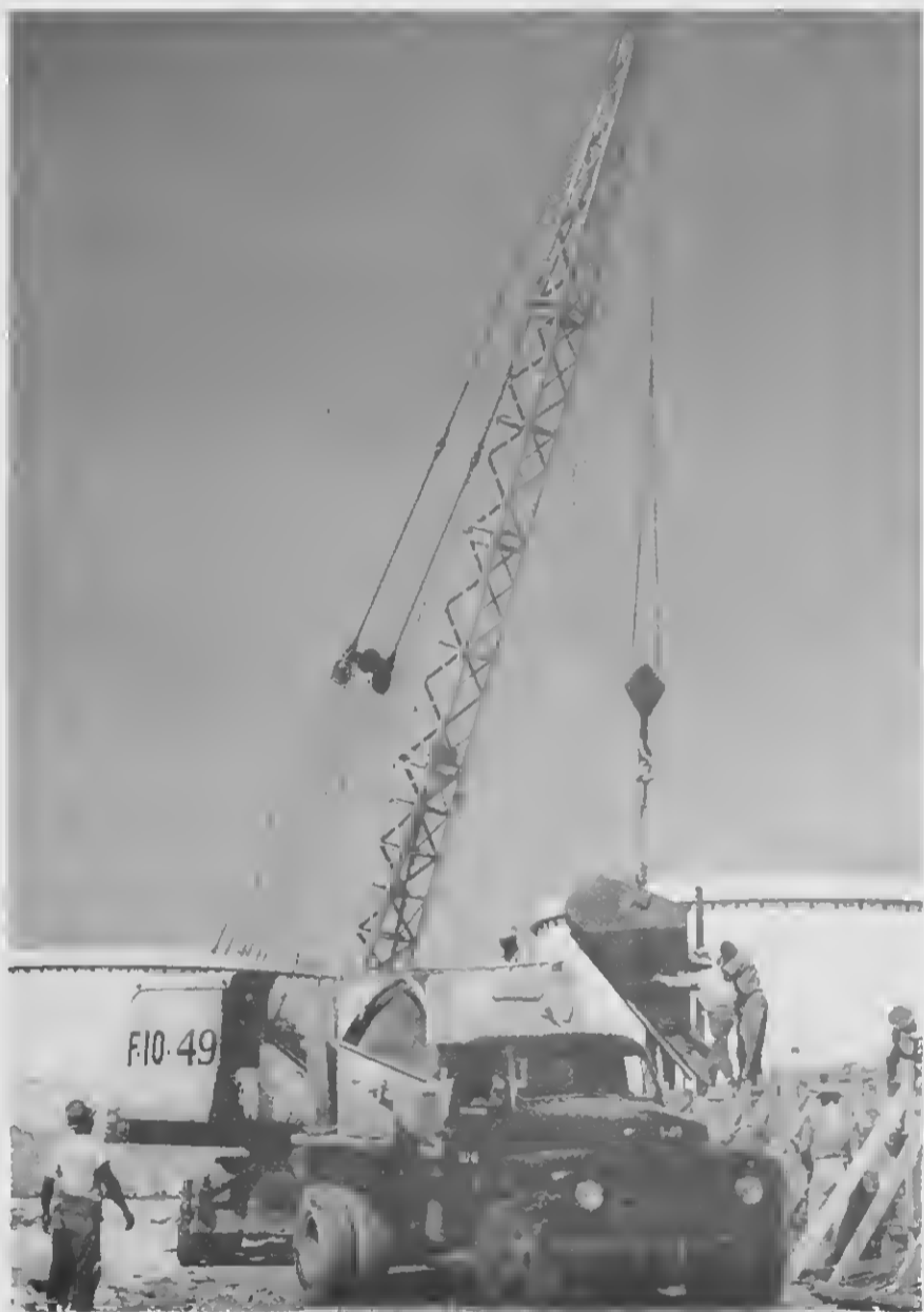
FOUNDATIONS ARE poured into the wooden forms. The concrete ring, when completed, stood eight feet high.
